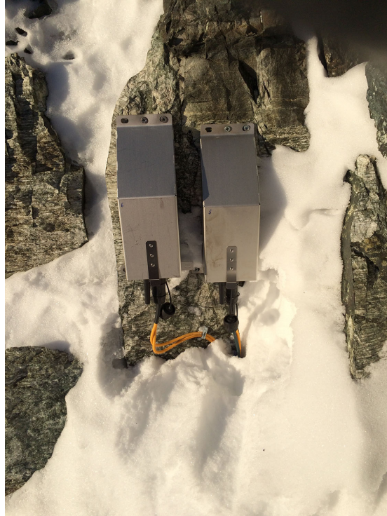
Figure C9. Sensor nodes at position MH05 and MH06 are installed on a small rock wall above a ledge to prevent heavy snow coverage while the sensors themselves are not visible.
