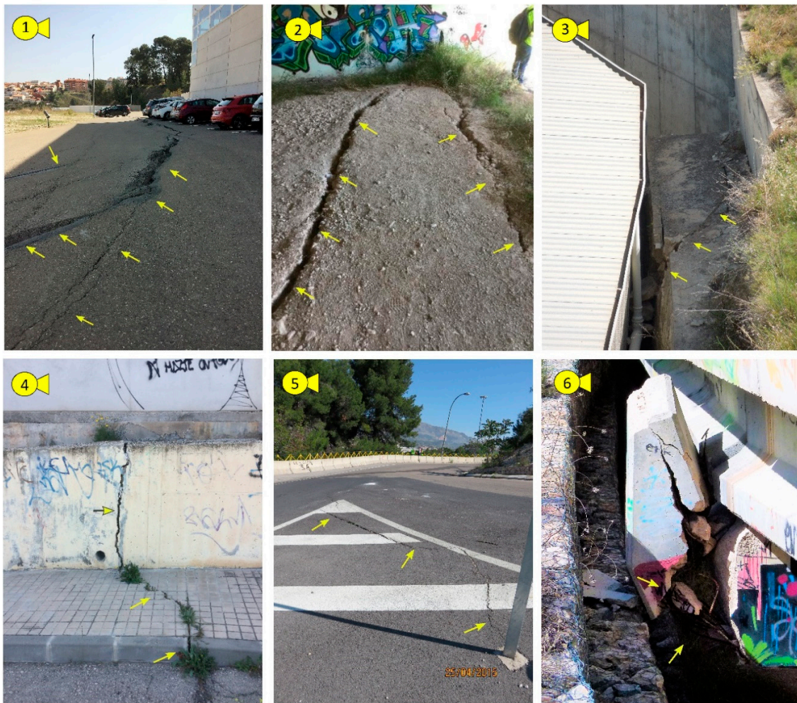
Figure 6. Photography of damages. (1) Crack at the head of the slope. (2) Crack on the soil surface beneath the bridge. (3) Broken wall at the bottom of the slope. (4) Cracked concrete fence located north of the bridge. (5) Crack on the pavement at the roundabout, north of the bridge and tilting of the lamppost. (6) Shear key broken because of precast beam lateral movement. Photos location are shown in Figure 1.
