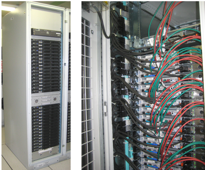
Figure 58. Left: front view of XPU rack (SDX Level 2) with 31 1U XPU machines, of which one is used only for monitoring and control, one local file server (at the top) and two “pizza box” concentrator switches (behind the panel in the middle), one connects to the Control Network, the other to the DataCollection as well as the BackEnd network (2.10.1). Right: cabling in the back of an XPU rack. The green and red cables are GbE cables connecting the nodes to the concentrator switches.
