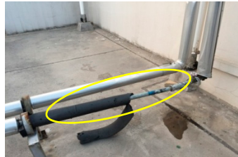
(b) Pipe insulation layer falling off
