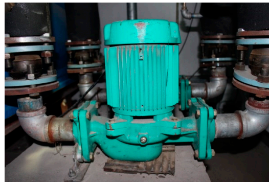
Figure 5. A circulating water pump without vibration reduction treatment.
