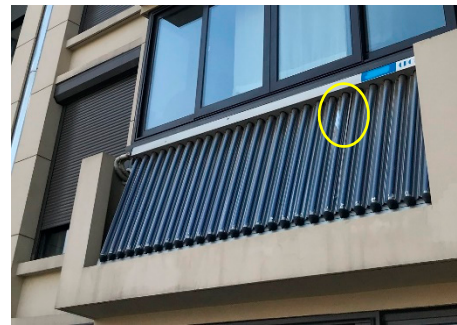
(b) One broken vacuum tube in a compound parabolic collector with a U-shaped copper pipe inside (CPC).
