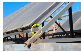
(c) The end nozzle is directly blocked, and scale is deposited.
