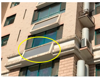
(a) No maintenance space.
