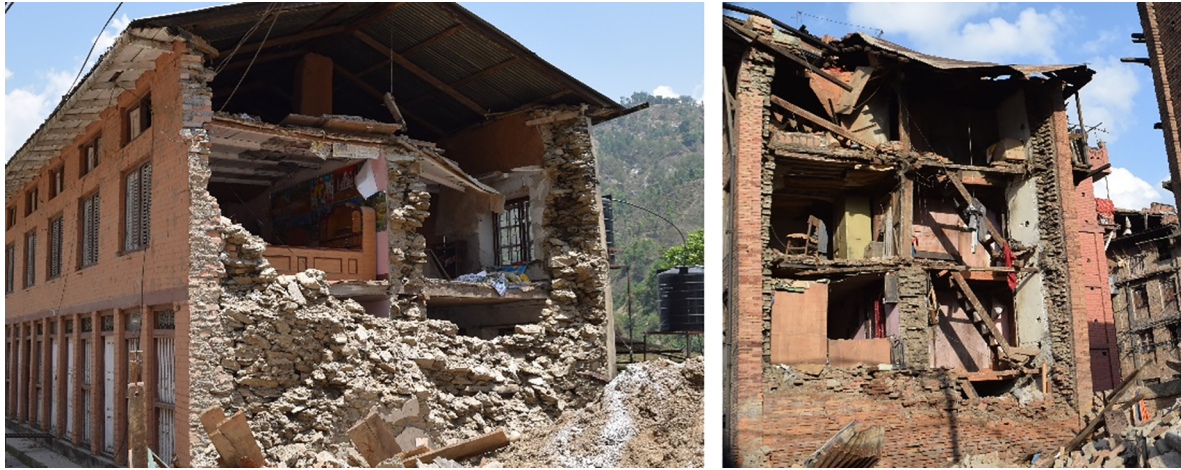
Fig. 1. OOP damage of Nepalese URM buildings (credits: Rama Mohan Pokhrel).
