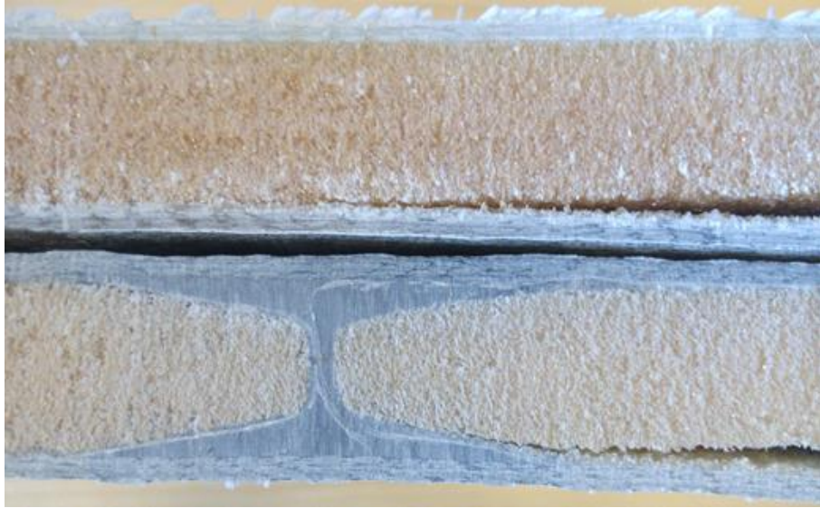
Figure 11. Post mortem sections of sandwich panel specimens PLT2 (above – no peel stopper) and PLP2 (below - with embedded peel stopper).
