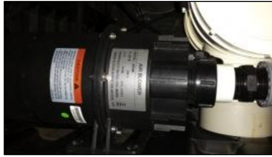
Figure 20: 200 watt air blower pump, used to assist backwashing.
