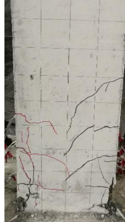
(c) Vertical crack
