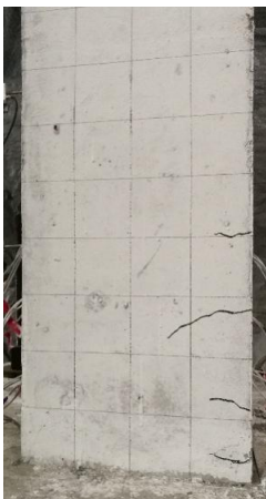
(a) Initial crack
