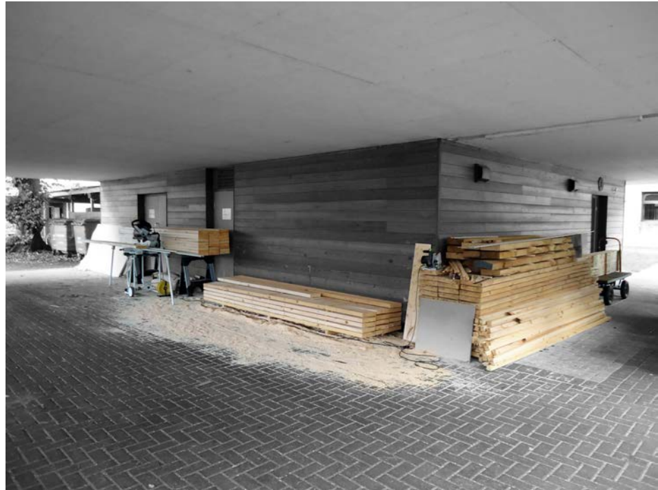
(a) Ripping and cutting individual boards to a consistent width of 200mm and a length of 2400mm, respectively.
