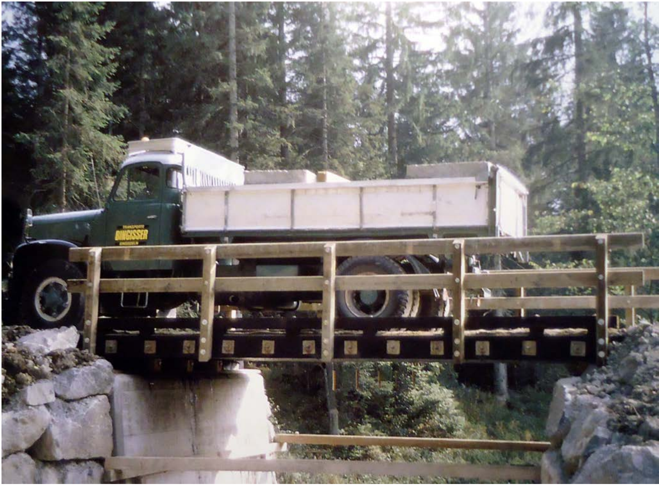
Figure 4.1: A stress-laminated bridge deck showing the bearing plates and ends of steel prestressing bars at the edge of the deck.
