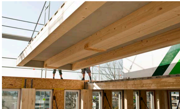
Figure 1.13(a) above and (b) below: Timber-concrete floor elements during assembly of the LifeCycle Tower One and Illwerke Zentrum Montafon buildings by Architekten Hermann Kaufmann ZT GmbH, 2012 and 2014, Dornbirn and Vandans, Austria. (Photographer: Darko Todorovic)
