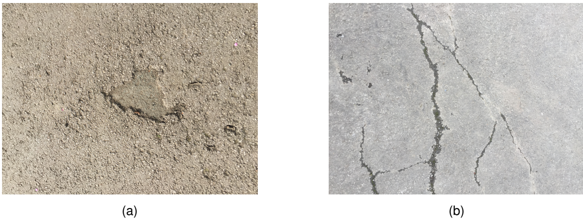
Figure 1: Original crack images from our dataset. (a) shows the first crack; (b) shows the second crack.
