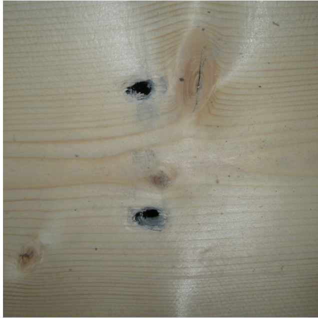
Figure 13: Typical local failure from embedment of the steel connector into softwood.
