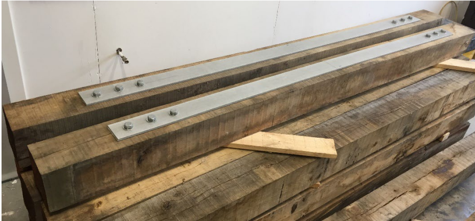
Figure 7: Hardwood beams reinforced according to screw configuration No. 2.
