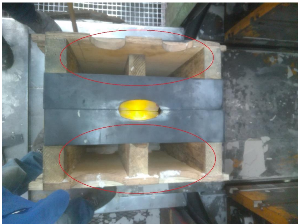
Figure 3.4 – Cavities that should be covered
