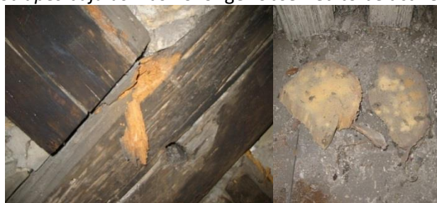
Figure 3: Left - Damage by Hylotrupes bajulus . Right - Sawdust of Anobium punctatum
