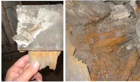
Figure 4: Left - Mycelium of the Dry Rot Fungus. Right –Brown Rot at the heading section of the beams
