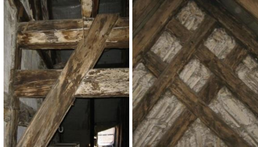
Figure 2: Left – Collar Beam Roof. Right – Wooden Stakes filling by Loam and Straw
