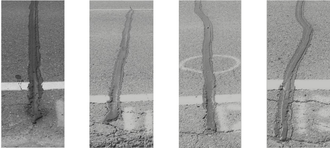
(a) Crack 10.5, 20x20 mm
