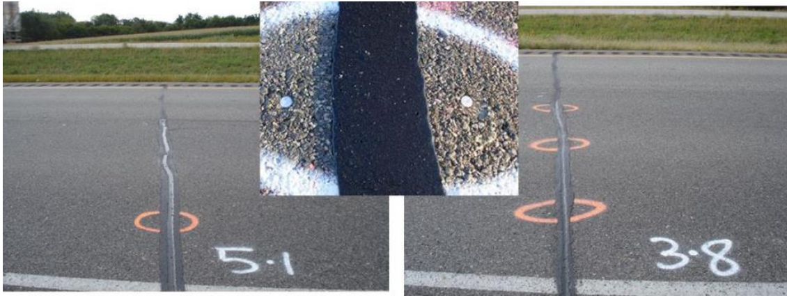
Figure 4.2. Crack displacement pins: Single-point measurement (left) and three-point measurement (right).
