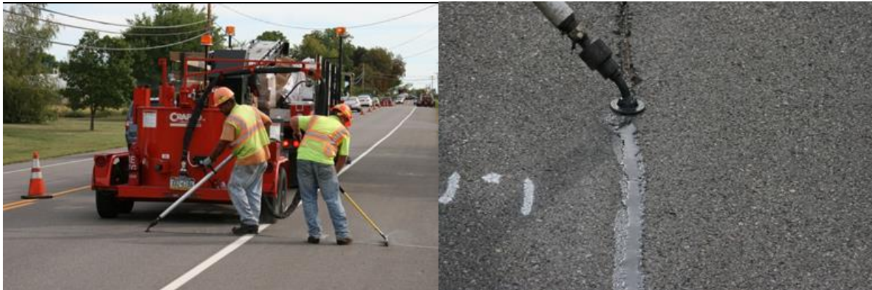
Figure 4.32. Kettle (left) and disk shape adapter (right) used at New York test section sealant installation.
