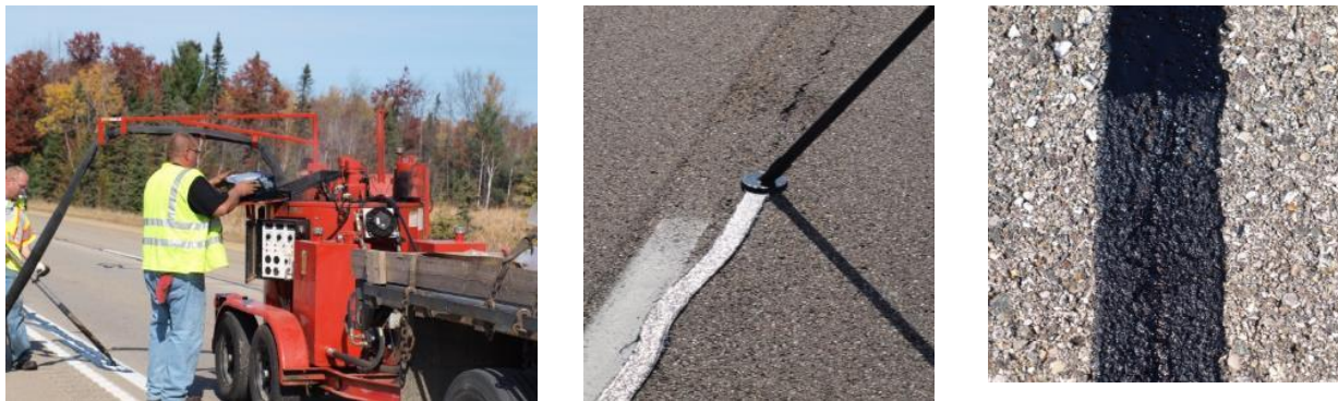
Figure 4.42. Typical crack filling operations: Heating the material in a kettle (left), sealant and overband application using disk adaptor (middle), and the finished product (right).
