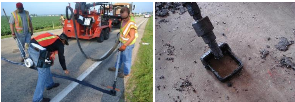
Figure 4.10. Kettle used in Wisconsin for heating sealant (left) and horse shoe adapter (right).
