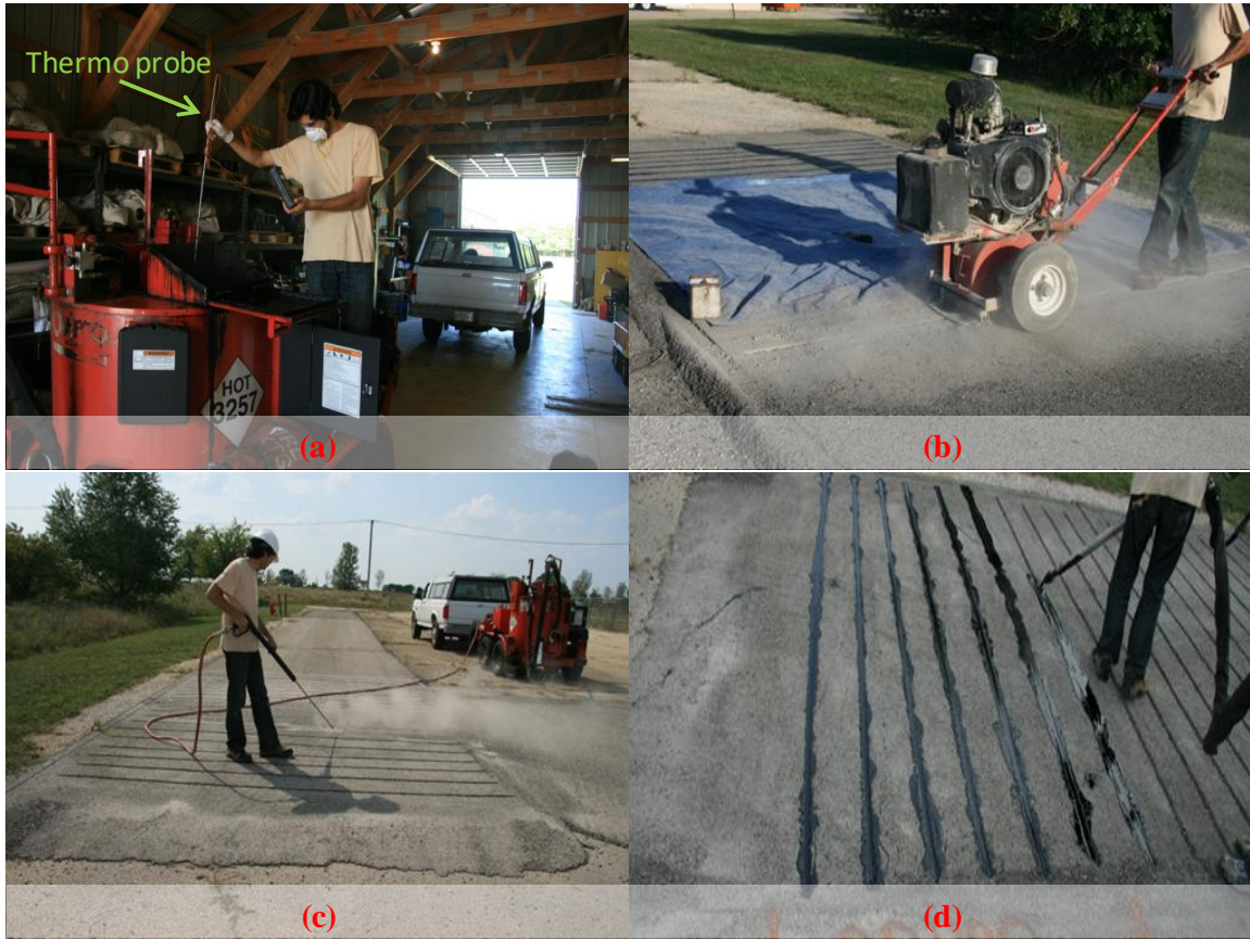
Figure 6.8. Sealant installation process: (a) Sealant heating and temperature monitoring; (b) routing; (c) rout cleaning with high-pressure air; and (d) finishing the installation in the routs.
