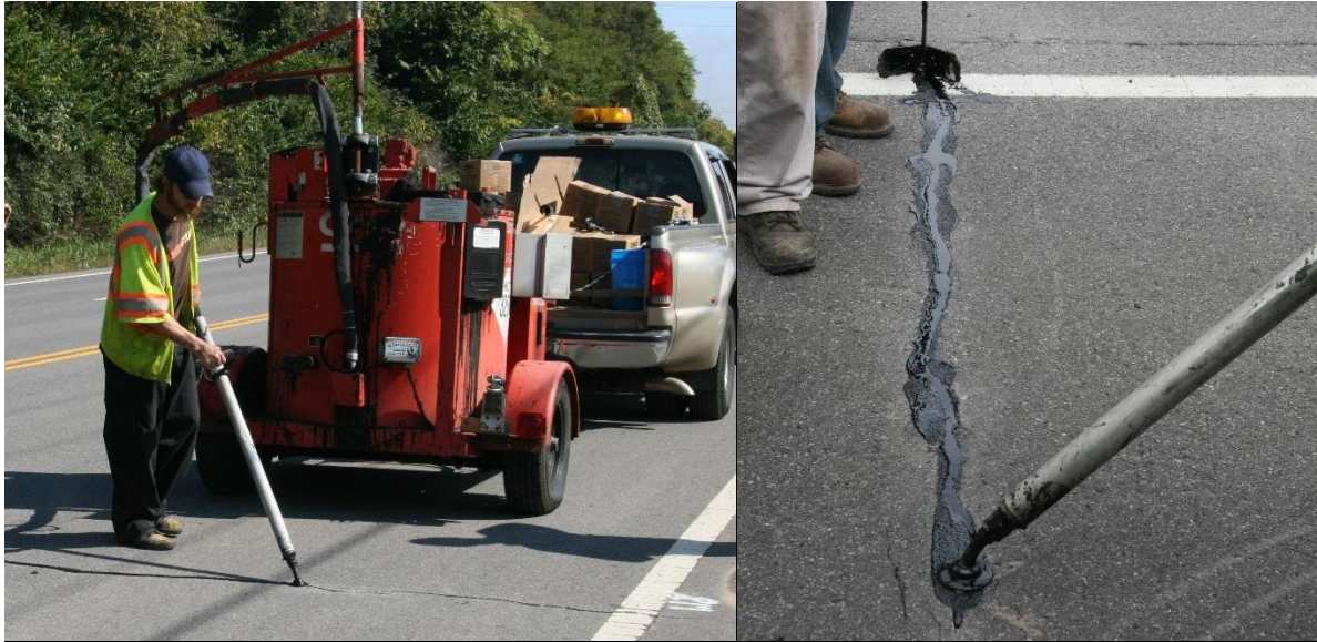
Figure 4.37. Kettle (left) and disk shape adapter (right) used at Virginia test section sealant installation.
