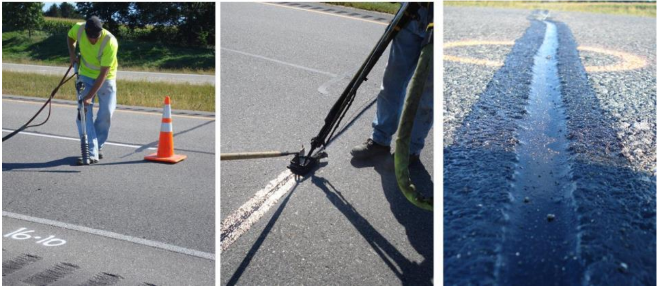
Figure 4.6. Typical crack sealing operations: Drying and cleaning the rout using hot air lance and compressed air (left); sealant and overband application using squeegee (middle); and the finished product (right).
