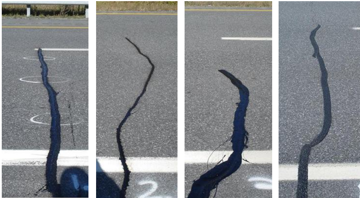
(a) Crack 1.8, 20x20 mm (b) Crack 2.6, 20x20 mm (no overband) (c) Crack 3.4, 20x20 mm (d) Crack 16.7, clean and seal Figure 4.28. Crack sealant treatment in Sections 1, 2, 3, and 16 in New Hampshire.
