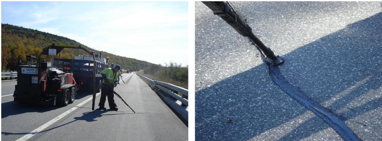
Figure 4.27. Kettle and sealant installation using disk shape adapter in New Hampshire. After draining the kettle to achieve kettle cleanliness, 300-400kg of sealant blocks were added to the kettle for each section. A time log detailing all activities is presented in Table 4.16. Sealant installation was completed in two days.
