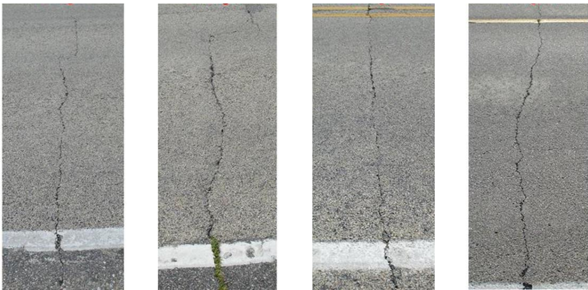
(a) Crack 1.1, Rating 4 (b) Crack 2.1, Rating 3 (c) Crack 3.25, Rating 4 (d) Crack 4.18, Rating 4.5
