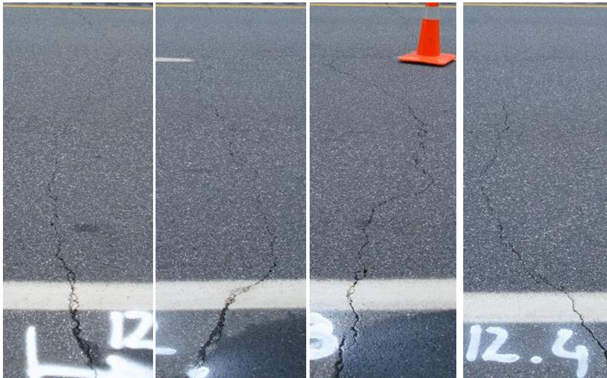
(a) Crack 12.1, Rating 4.5 (a) Crack 12.2, Rating 5 (a) Crack 12.3, Rating 4 (a) Crack 12.4, Rating 5 Figure 4.26. Initial crack condition in Section 12 of the New Hampshire test site.
