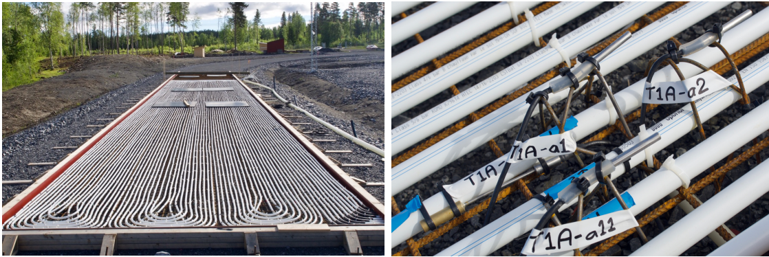
(a) Pipe in the HHP.
