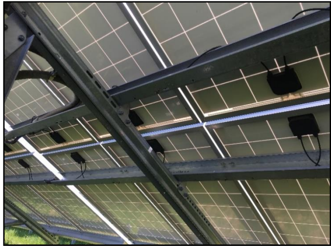
Figure 5. Support structure under solar panels
