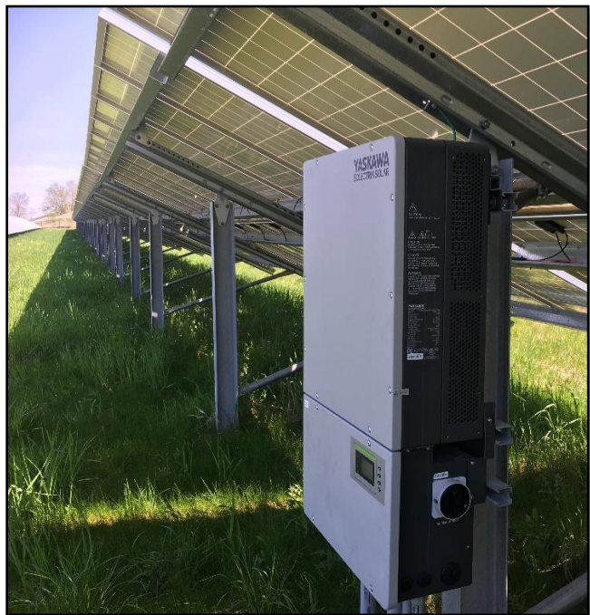
Figure 6. One CFU solar panel inverter
