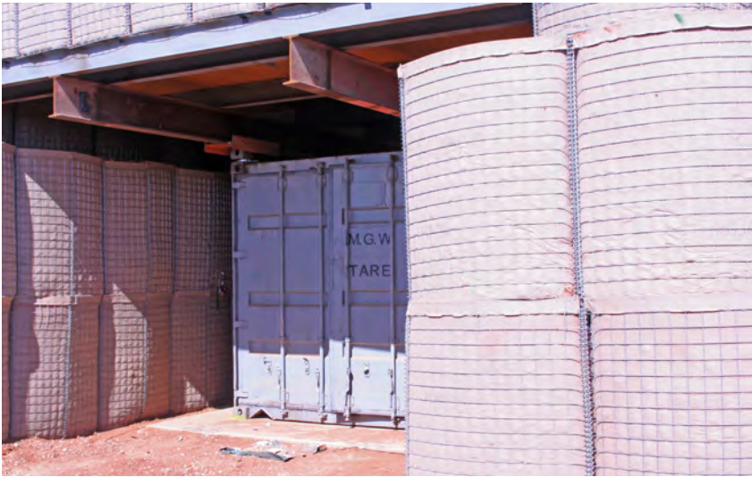
Figure 20 – Shipping Container Based Magazine with Overhead Protection. 100)
