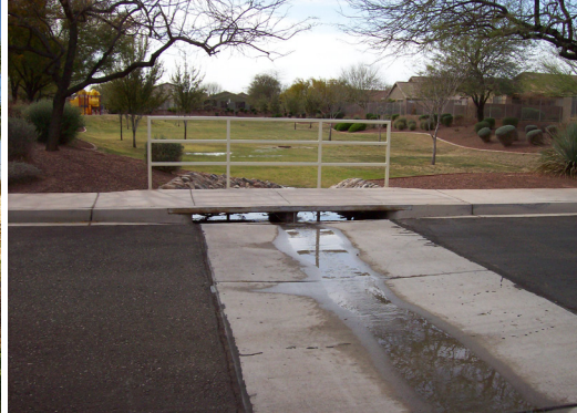
Stormwater Outlet and Green Infrastructure
