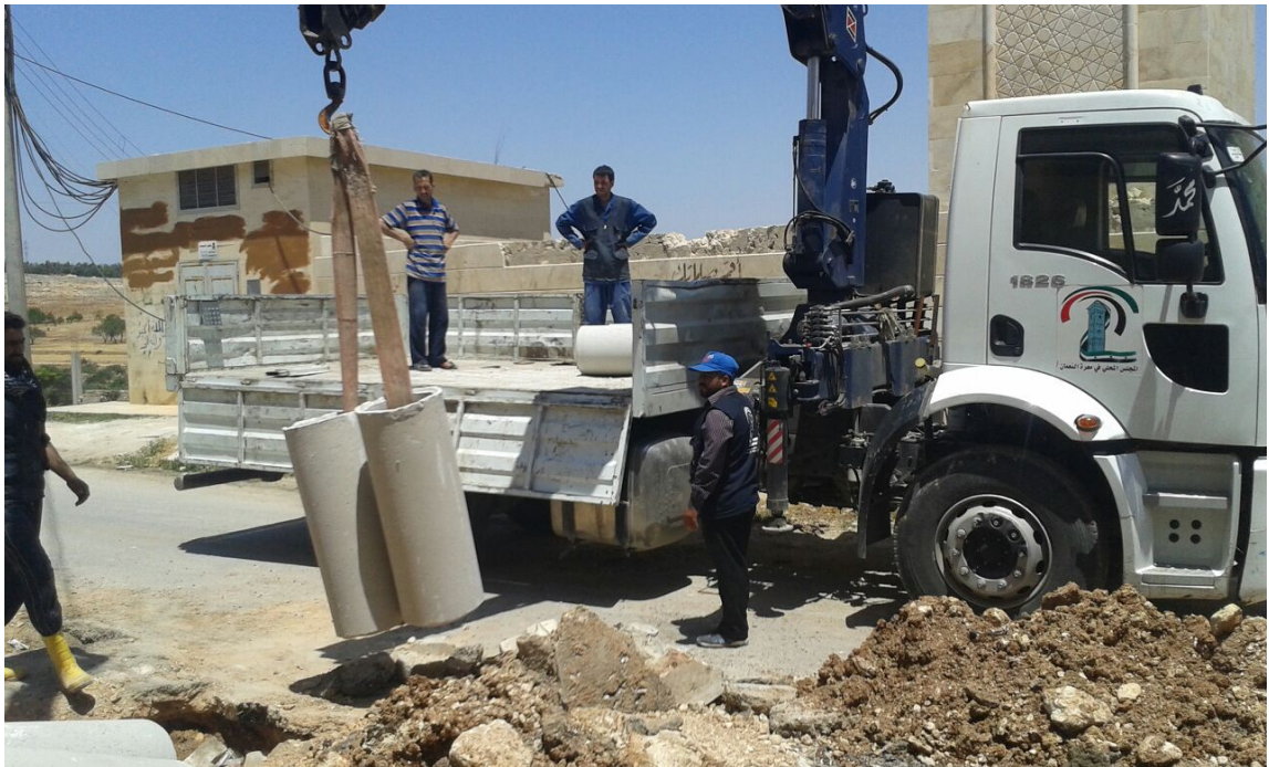
Figure 8 Photo posted by the Local Council of Ma'arat a-Nu'man on June 7, 2016 of men doing repairs
