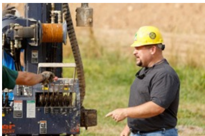
Mike Malusis, Professor of Civil and Environmental Engineering, supervises construction efforts at the new slurry wall facility at Montandon Marsh. [Photo by Brett Simpson, Bucknell Division of Communications]
