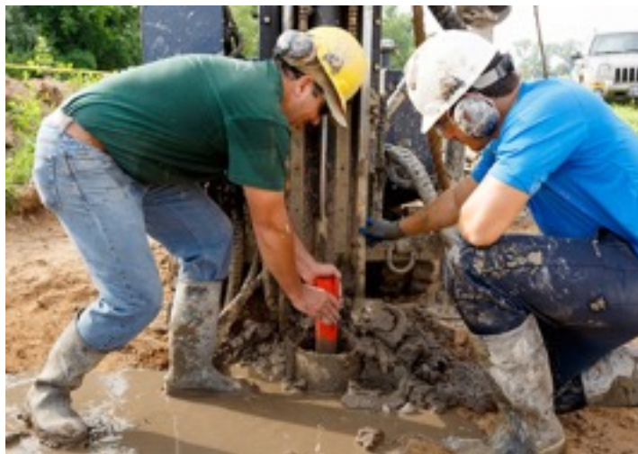
James Gutelius, director of Civil Engineering labs, (left) oversaw drilling and installation of groundwater monitoring wells around the new slurry wall facility at Montandon Marsh. [Photo by Brett Simpson, Bucknell Division of Communications]
