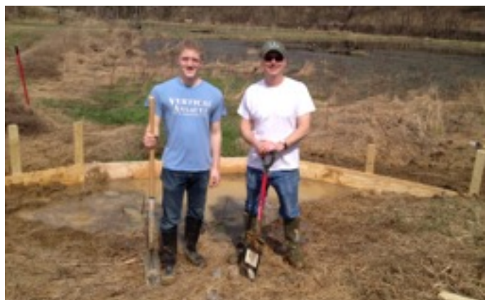
Civil and Environmental Engineering student Gareth Messman '17 and Professor Matthew Higgins helped install a v-notch weir to measure flow into one of the agricultural treatment wetlands installed at Ards Farm in Lewisburg, PA. [Photo by Benjamin Hayes]
