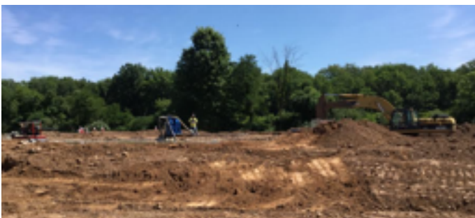
The new slurry wall being installed. Bentonite mixer visible on left and backhoe digging the trench on right. [Photo by Sean Reese]
