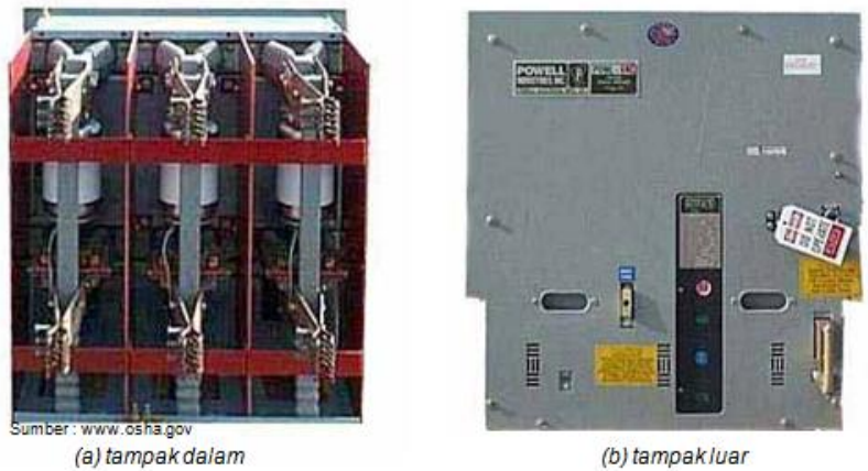
Gambar 2.15 VCB (Vacum Circuit Breaker)
