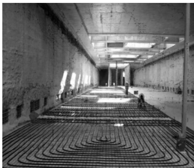
Figure 2.4: Absorber pipes deployed above the floor slab of the U2 Messe-Prater metro station (Vienna, Austria). From Adam and Markiewicz (2009)
