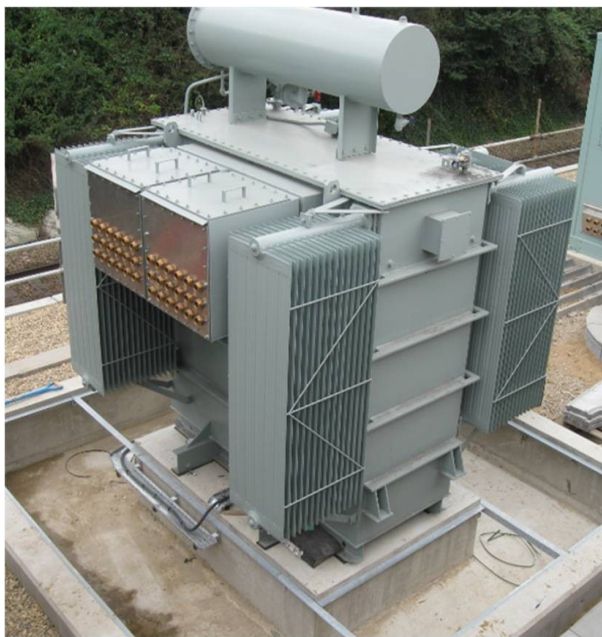
Fig. 1. Transformer in its Final Location with arrangements made for bonding, prior to the installation of the rain shelter.
