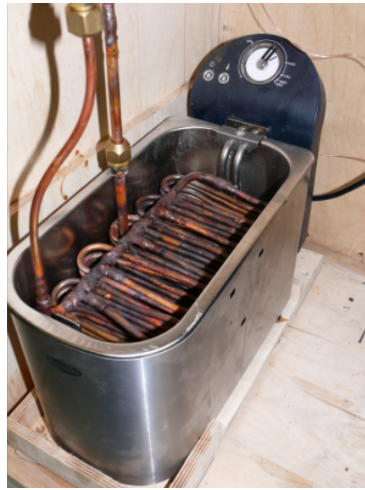
Figure 5.18: Photograph of generator heat exchanger EP1 - Version 1
