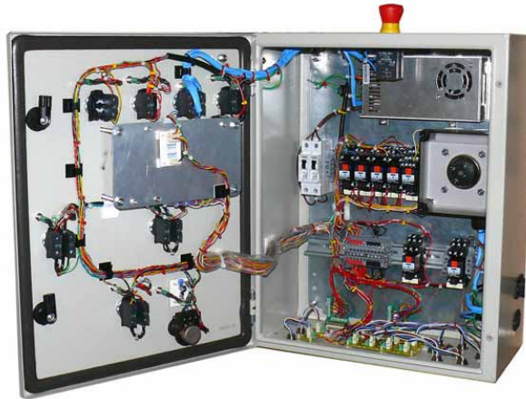
Figure 6.24: Photo of control box
