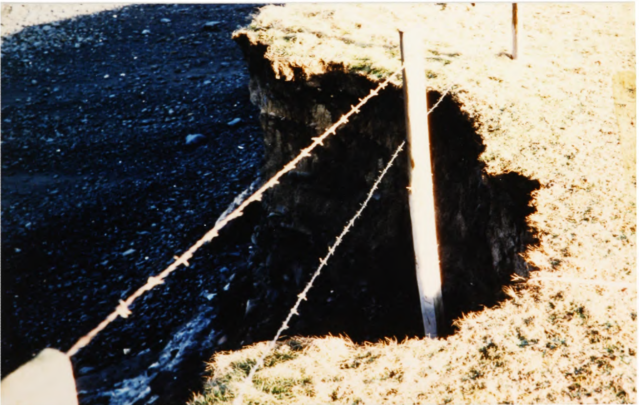
PLATE 3.14 View from cliff top of individual failure at chng. 89 + 50 ( 14.4.84 )
