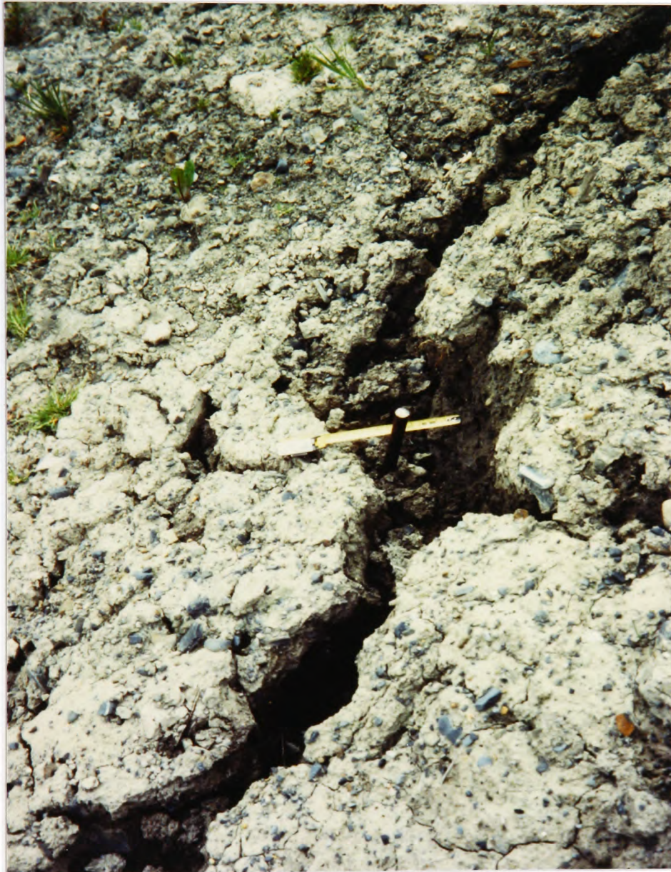
PLATE 9.12 Desiccation cracks in clay slopes at New Quay. Aug '84
