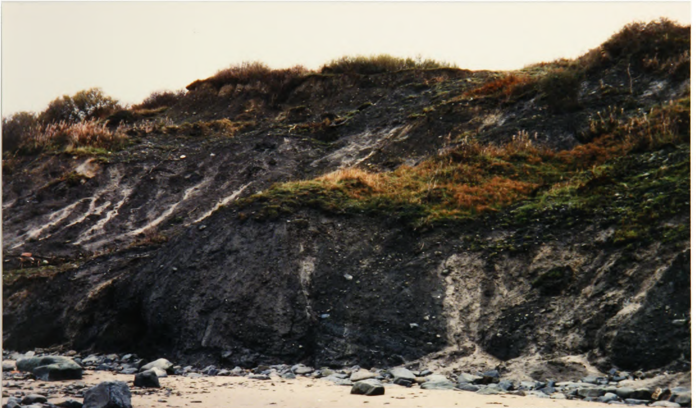
PLATE 9. 11 Sub-aerial erosion of boulder clay slopes at New Quay
