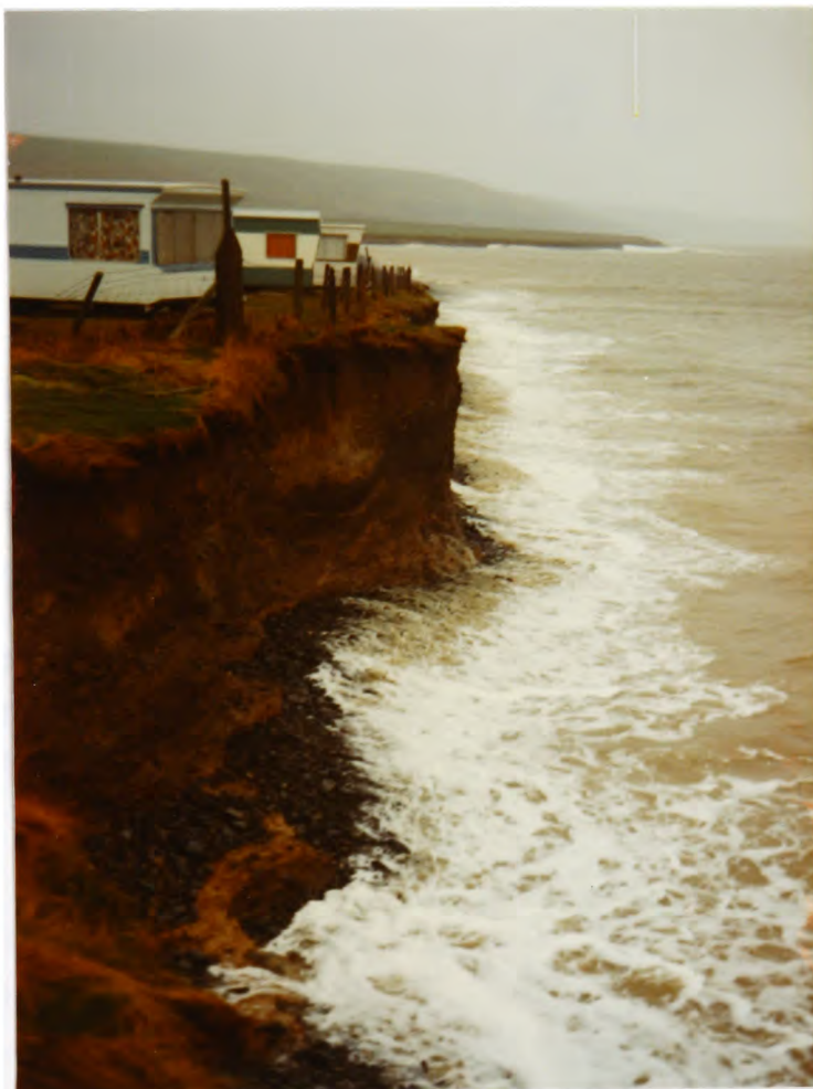
PLATE 4.3 Erosion of cliff base at Llanon (3.1.84)
