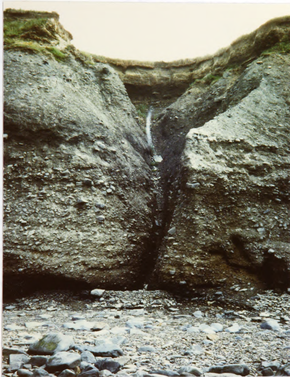
PLATE 9.9 Extensive gullying of till material chng. 80 + 00 approx.
