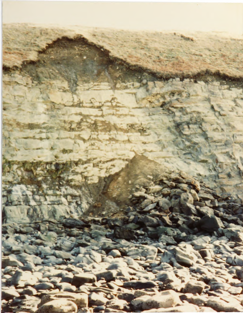
PLATE 9.3 · Rockfall near Graig Ddu (Mar 1984)
