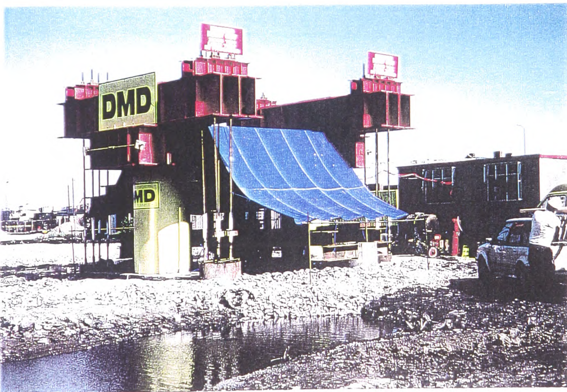
Plate 3.7 A 2000 ton test loading rig developed by DMD Piling Ltd (Cardiff) utilising 4 anchor piles
