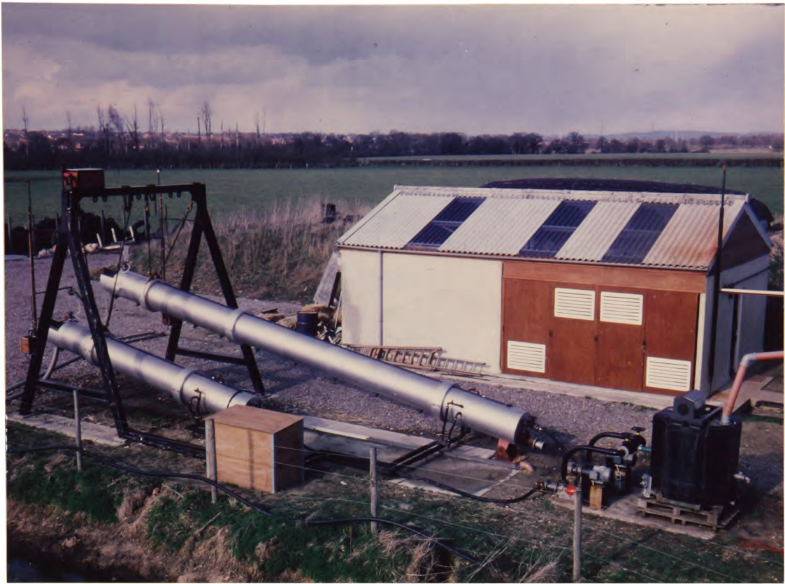
PLATE 1. Pilot scale inclined tubular digesters.
