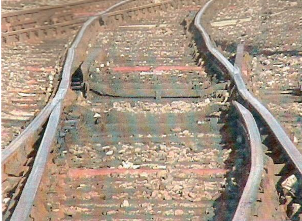
Figure 5: Poor Alignment due to Insufficient Maintenance Erewash Valley 1997(Source: author)
