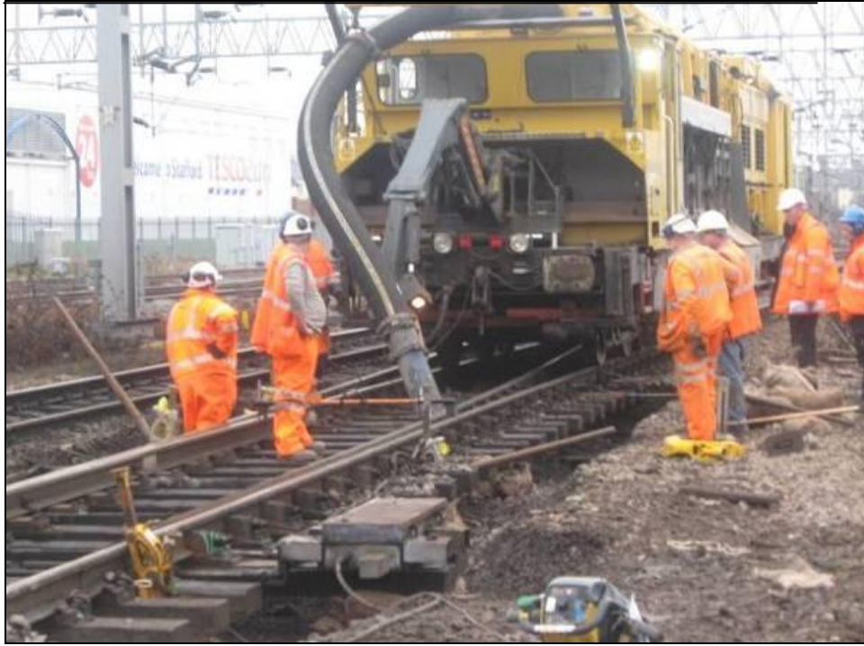
Figure 44: Use of Railvac in adjacent areas to ramp in new work (Source: Sersa-UK Ltd.)
