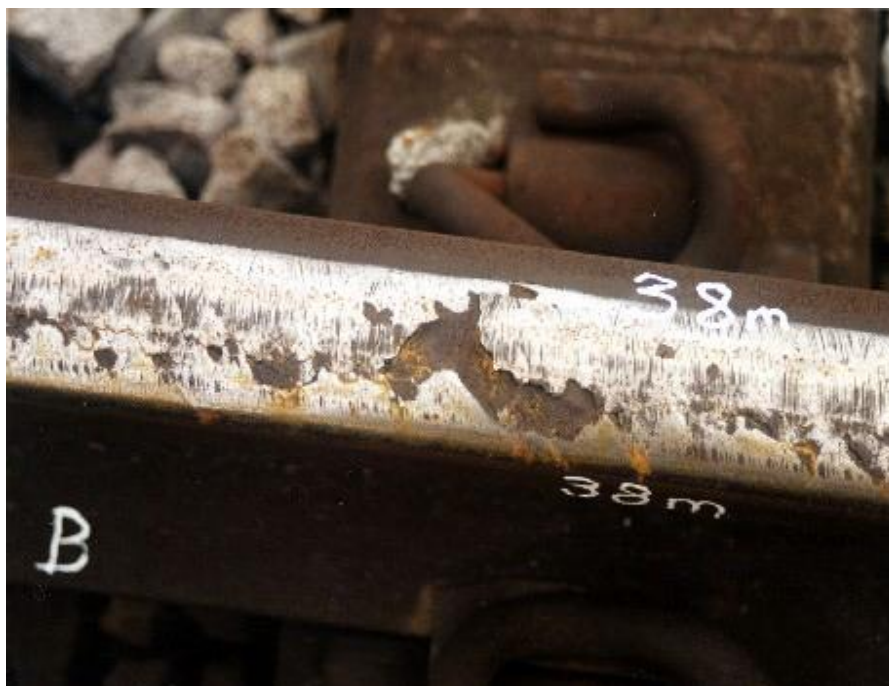
Picture of railhead close to the Hatfield site where transverse fatigue cracking can be seen and the initiation of severe spalling. Source: ORR 2002
