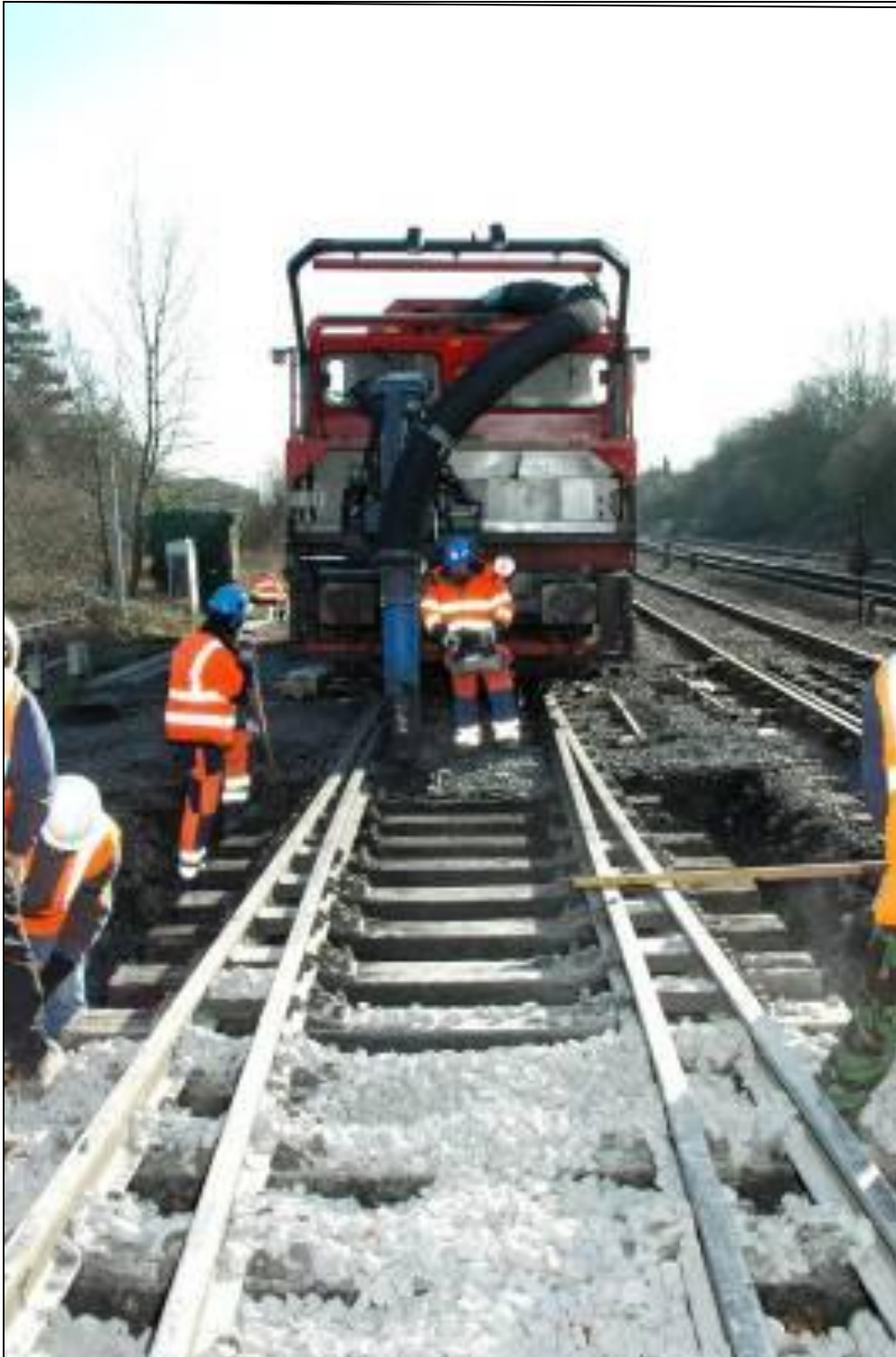
Figure 20: Railvac vacuum reballasting machine showing excavation Switch and crossing layout at Foxhall Junction, Didcot, UK. (courtesy Railcare)
