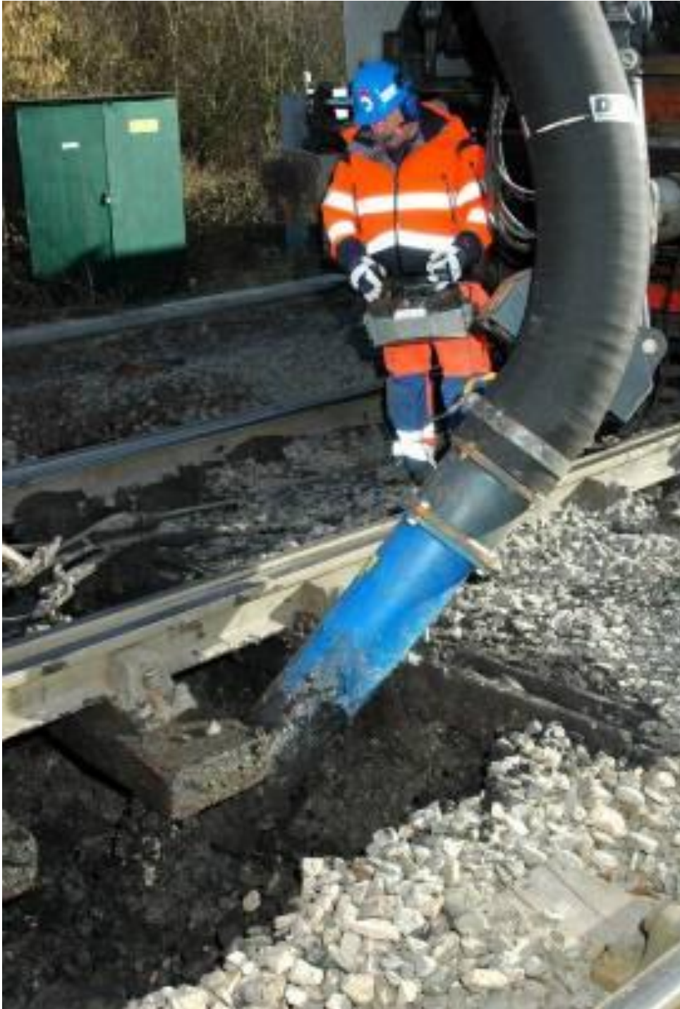
Figure 19: Railvac vacuum rebalasting machine showing tungsten tube Switch and crossing layout at Foxhall Junction, Didcot, UK. (courtesy Railcare)
