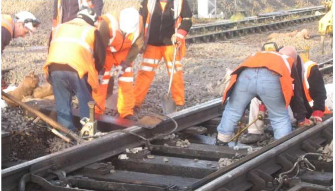
Figure 33: Changing Switch and Crossing timbers on the West Coast Main Line (Source: author)
