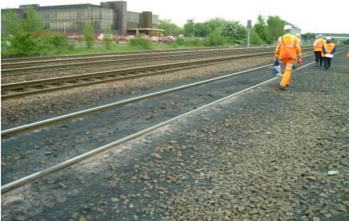
Figure 35: Spillage of coal choking the ballast and covering the track Wrawby Junction (Source: author)
