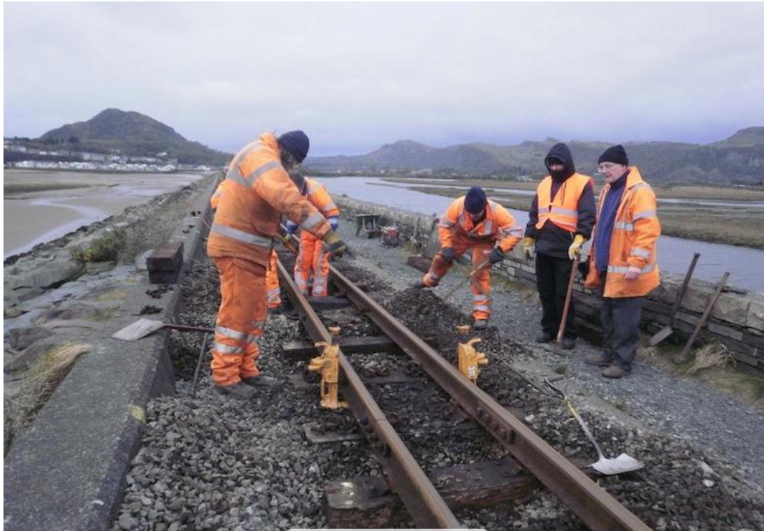
Figure 2: Patch re-sleeping on the Ffestiniog Railway at Porthmadog, Wales, UK, 2013 (courtesy: Ffestiniog Railway Ltd.)
