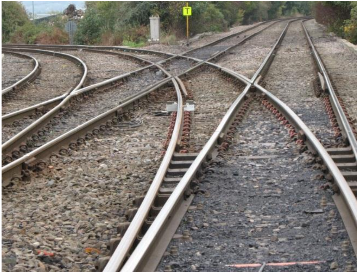
Figure 16: Railvac Re-Ballast and Refurbish Double Junction at Meadow Lane Trent UK 2010 (Source: author)
