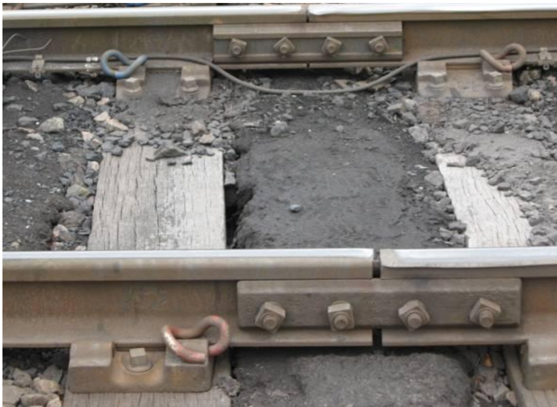
Figure 38: Wrawby Junction Severe Contamination at a rail joint (Source: author)
