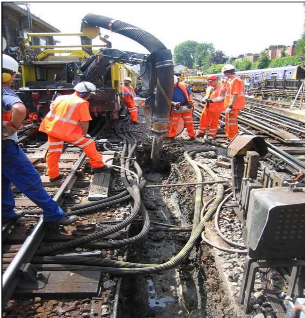
Figure 1: Railvac in a complicated track area with extensive cabling (Source: London Underground)
