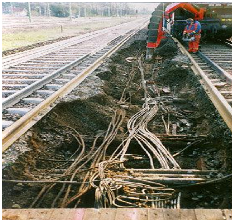
Figure 48: Railvac excavating in a track area with complex buried cabling (Source: Railcare SE)
