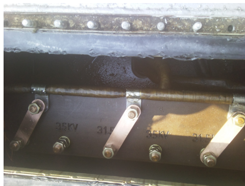
Fig. 11. A photo of loose connection failure for the TR-2 in the repair service
