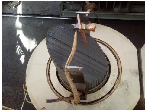
Fig. 10. A photo of faulty part of the TR-1 in the repair service
