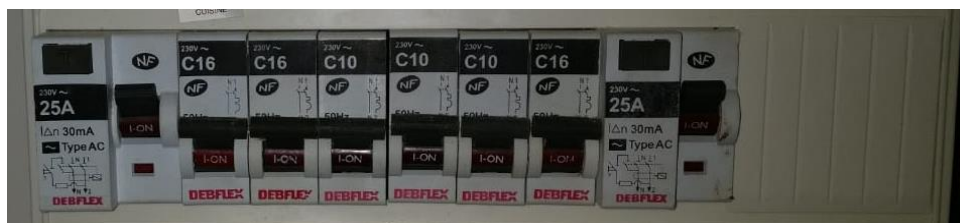
Figure 4.2 AC panel of the installation, with two RCDs at each end and six circuit-breakers (one of which is unused).
