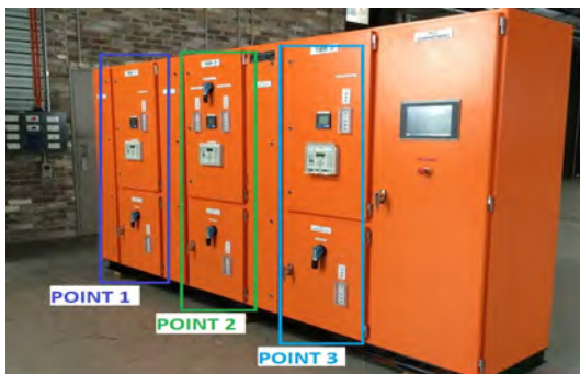
Fig. 6. Microgrid plug and play connection panel.
