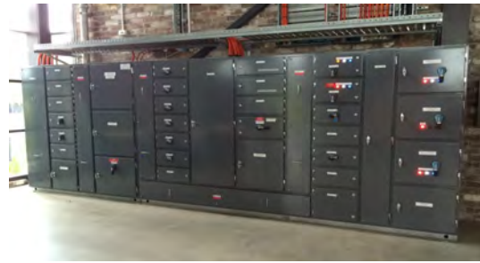
Fig. 2. Microgrid switch board (MGB) of laboratory microgrid.
