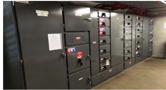
Fig. 3. Main switch board (MSB) of laboratory microgrid.
