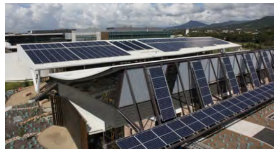
Fig. 4. SBRC photovoltaic system.
