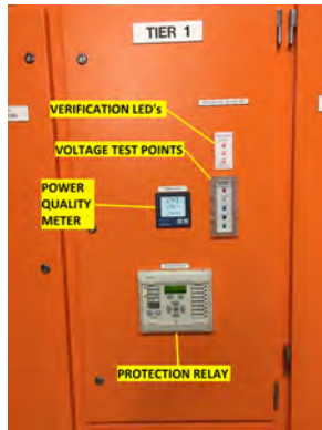
Fig. 10. Connection panel protection relay, power meter and test points.
