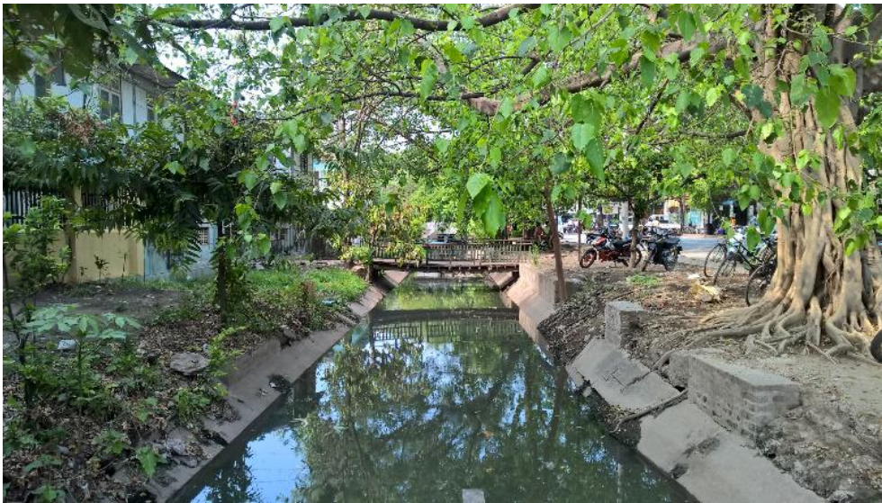
Figure 5. Precast drain in Maha Aung Myay. Source: J.Sanchez
