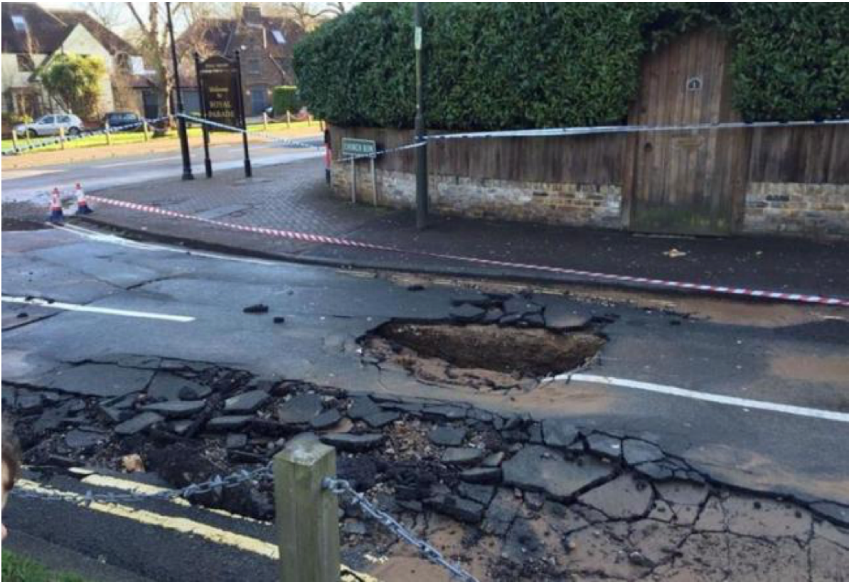
Fig. 3.17 Disruptive event cause
