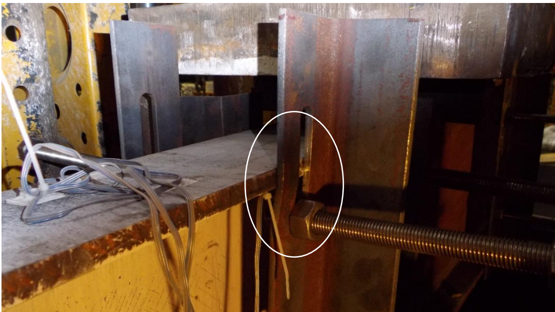
Figure 5.3.15: Local deformation in a bracing angle
