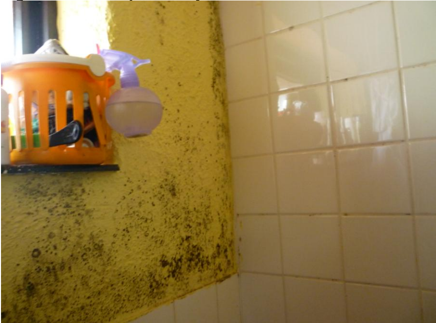
Figure 4.5.4 Damp in utility block
