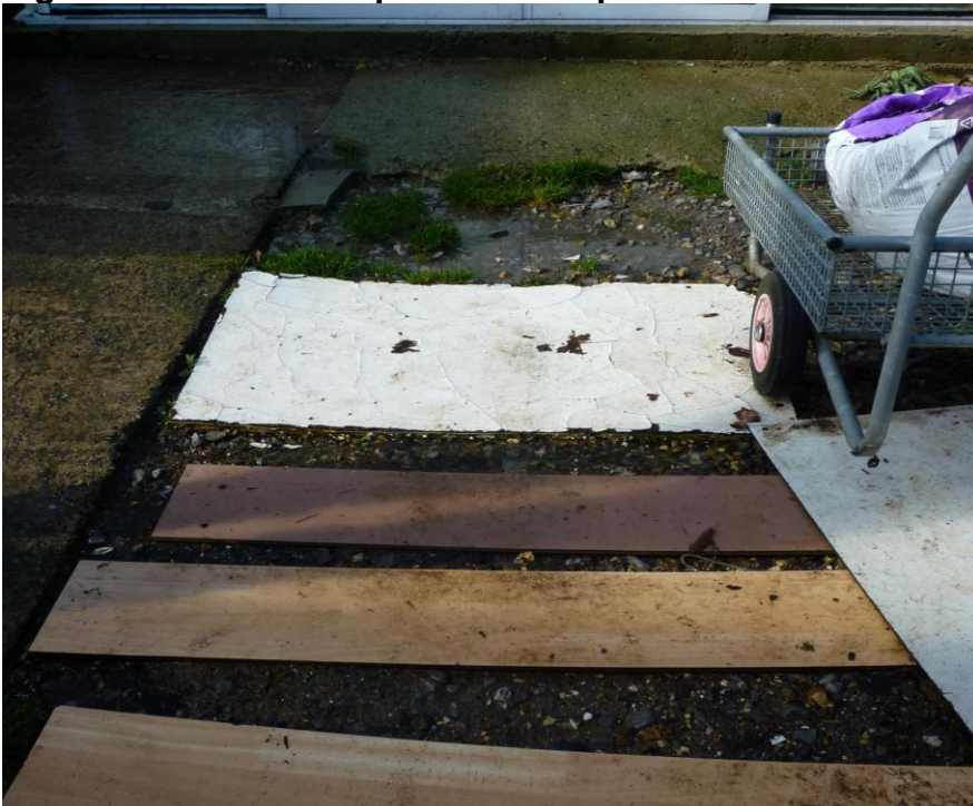
Figure 4.5.5 Concrete pitch in disrepair
