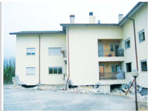
Figure 2. Soft story fracture due to elimination of masonry infill wall in ground floor in the 2006 L'Aquila earthquake [26]
