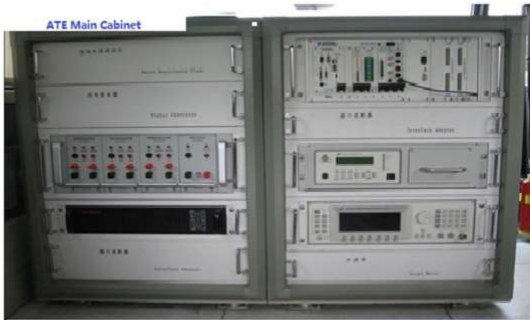
Figure 9 ATE Main Cabinet
