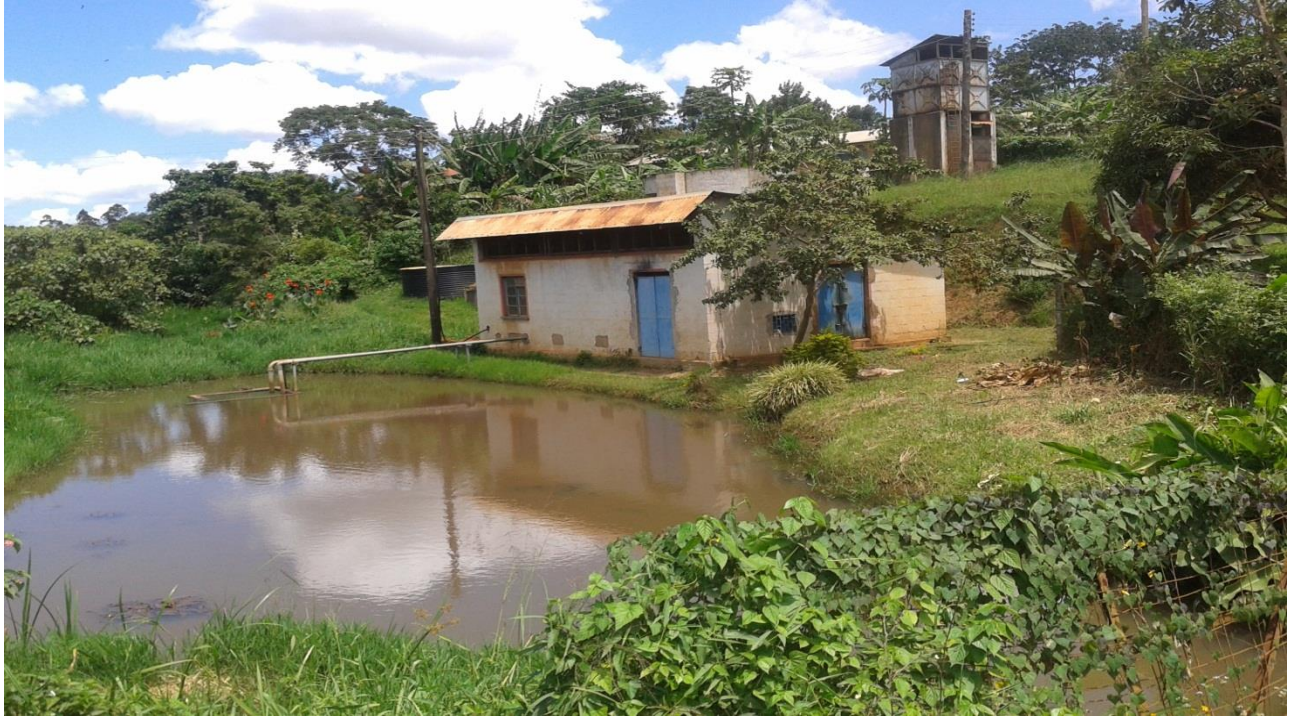
Figure 6.7: Filtration / flocculation facility in Lwajjali wetland – KMC.
