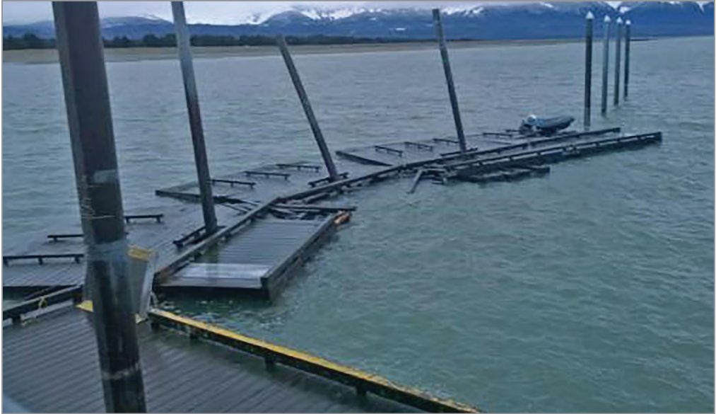
Damaged Boat Ramp (Canfield, 2014)
