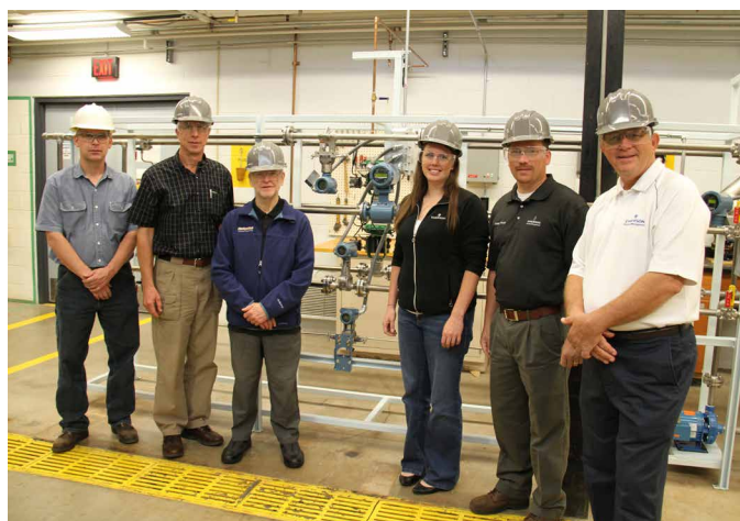
The new Flow Measurement and Control Experiment was commissioned on October 4, 2011. L to R: Jerry Norkol, Dave Caspary, Dr. Tony Rogers, Casey Hanlon, Terry Worm and Dennis Bialecki.
