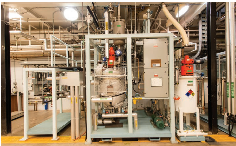
The solvent recovery unit, a three-story distillation column in the UO Lab
