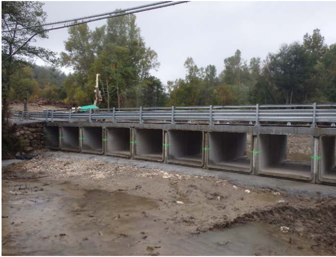
Figure 12. Temporary bridge bypassing the Ponte a Tre Occhi in Amatrice (Mr. Totaro, personal communication).
