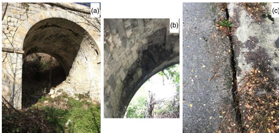
Figure 5. Roman-era bridge along the Trisungo route (1 span bridge, Tufo area, Arquata del Tronto: 42.7360 deg, 13.2549 deg): (a) View of the arch following the October event; (b) spalling of the interior of the arch; and (c) road cracks after the 24 August event, which grew slightly during the October event
