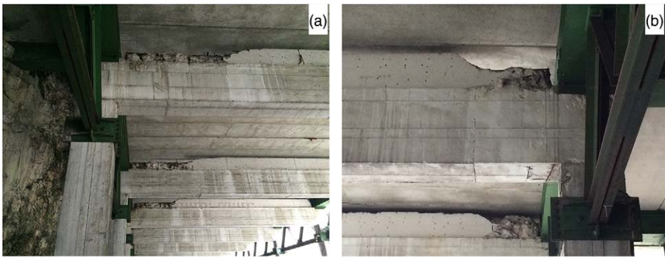
Figure 11. (a, b) Close-up views of reinforced concrete beam-column joint and the steel frame.
