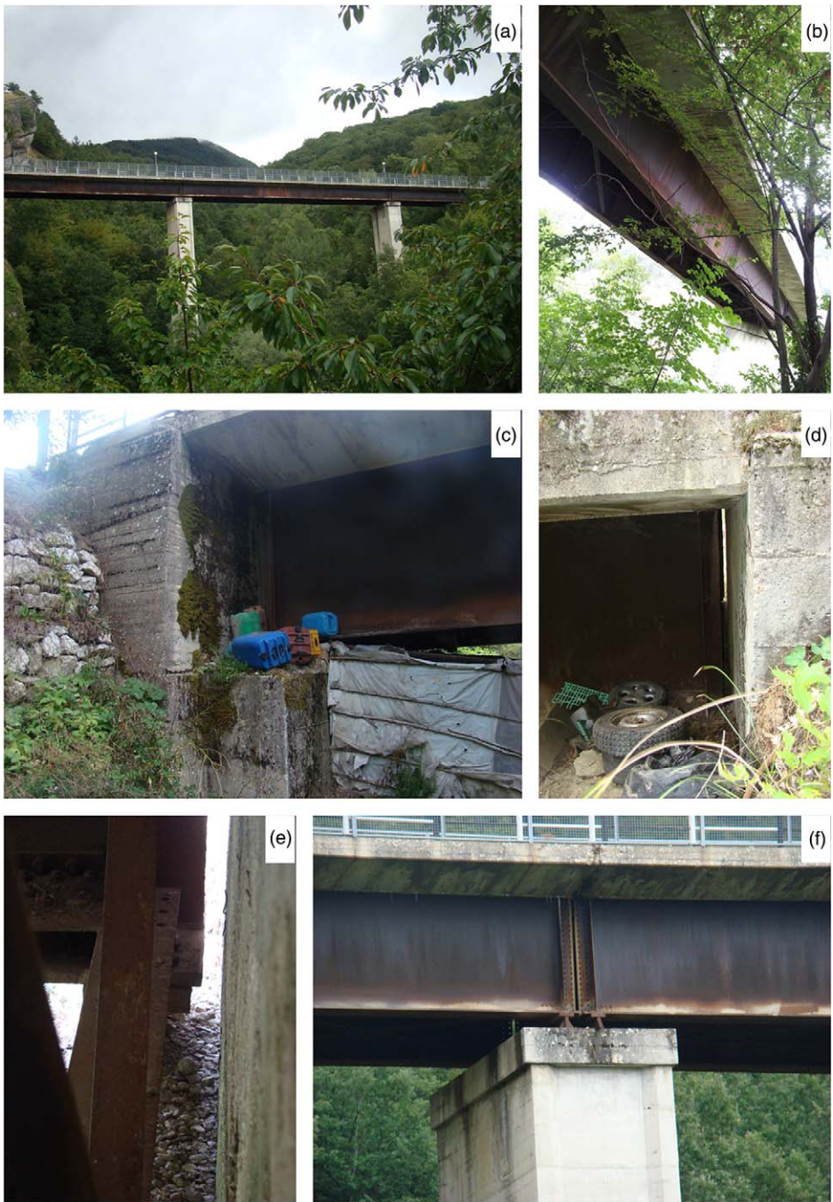
Figure 3. Ponte Ramazzotti : Composite steel and concrete bridge along the SP20 in Colle (42.7276 deg, 13.3111 deg). (a, b) overview of the bridge, (c) abutment, and (d, e, f) bridge support details.
