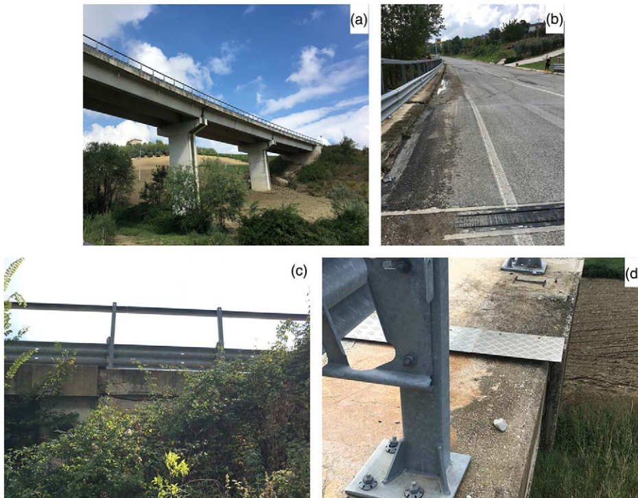
Figure 4. RC bridge along the SP173 in Offida (42.9417 deg, 13.7023 deg): (a) Overview of the bridge; (b) settlement of the road; (c) crack; and (d) relative displacement of the abutment.
