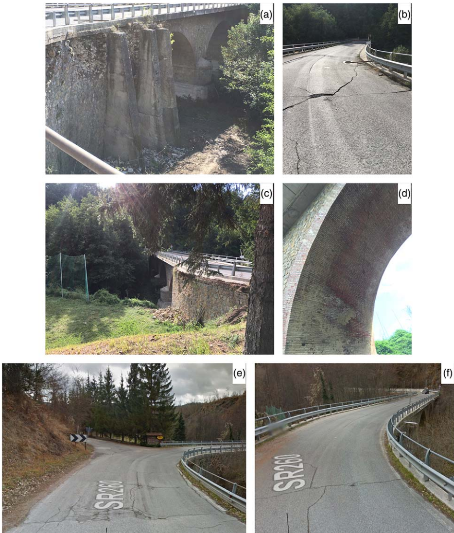
Figure 8. Ponte a Tre Occhi : Masonry bridge along the SR260 in Amatrice (42.6207 deg, 13.2902 deg). (a, c) Abutment deformations on two sides of the bridge, (b) road settlement, (d) cracks on the arch, (e) pre-event cracks along the SR260, and (f) bridge–abutment connection [source for (e, f): Google Maps ( https://www.google.com/maps/ ; last accessed 13 September 2018)].
