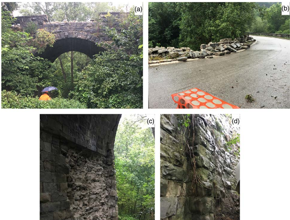
Figure 6. Central arch of the Roman-era three arches masonry bridge along the Trisungo route (42.7354 deg, 13.2537 deg) as observed following the August 2016 event: (a, b) Partial collapse of the railing; (c) spalling; and (d) cracking of some masonry elements in the central arch.
