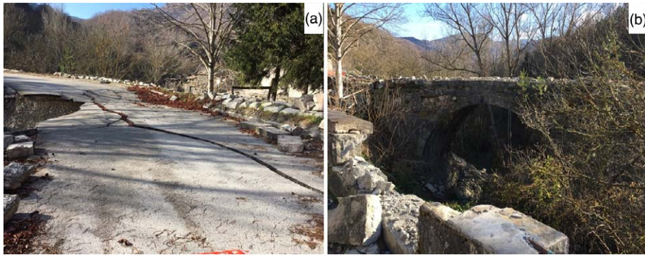
Figure 7. Three-arches bridge along the Trisungo route (same location as in Figure 6) after the 30 October 2016 event (photos taken on 13 December 2016). (a) Large longitudinal cracks on the roadway surface (same location as Figure 6b); and (b) total collapse of the masonry rail (same location as Figure 6a). The collapse of the arch is not visible in the pictures.
