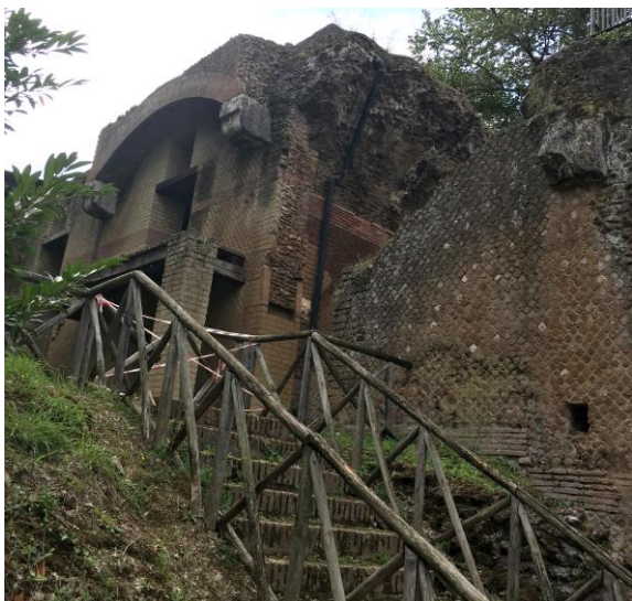
Fig. 14: Hadrian's Villa, western substructure of the Serapeum-Canopus, so-called Tabernae , collapsed vault. Image credits: A. Ottati
