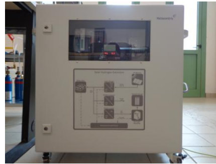
Power management cabinet
