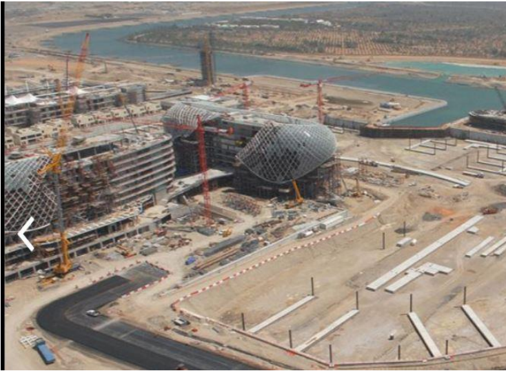
Figure1: Yas Marina F1 motor racing construction site – Yas hotel and its grid shell
