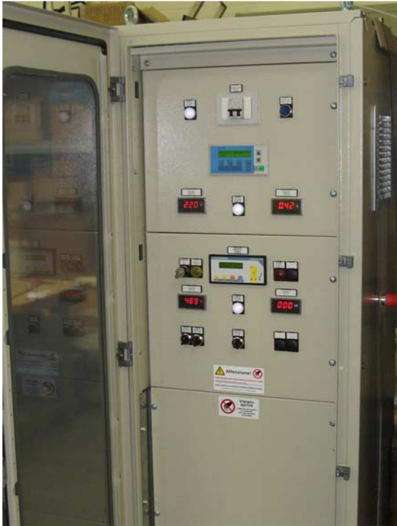
Fig. 12. Photo of the power supply rack installed at the shore station to power the SN1 abyssal station.
