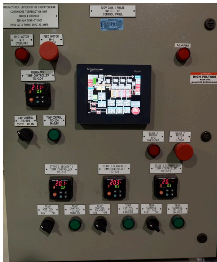
Figure A.3.9: CTU Control Panel
