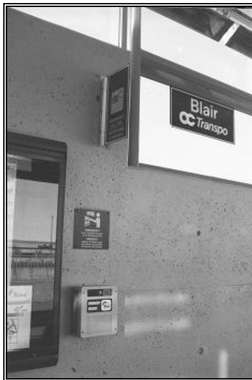
Figure 4.8 Emergency Call Box at Transit Station, Ottawa Photo: C. Fullerton
