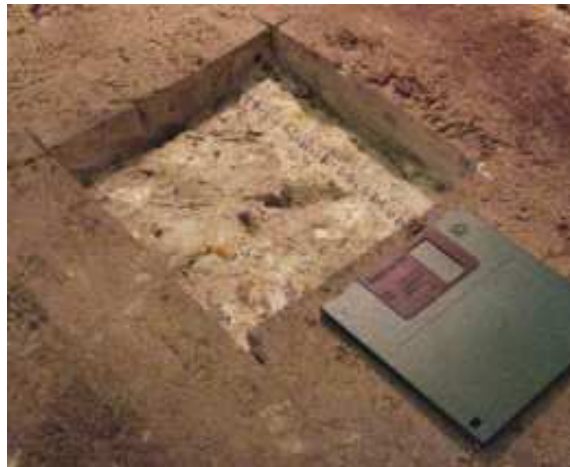
Figure 5.18. Experimental damage induced on the surface of the girder.
