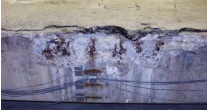
Figure 6.26. The deteriorated vertical surface of the girder near a stain gauge installation.
