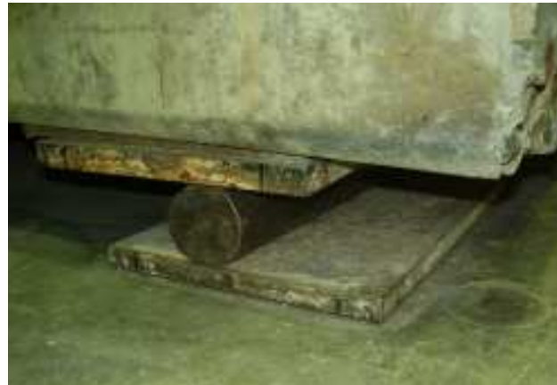
Figure 5.17. Photographs of the supports of the girder: (a) steel angle support at one end of the girder, and (b) roller support at the other end.
