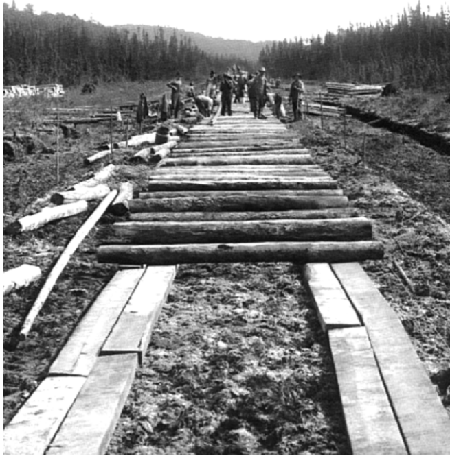
Figure 6.3 : Photograph of the construction of a railway embankment over peat using corduroy raft construction (MacFarlane 1969).
