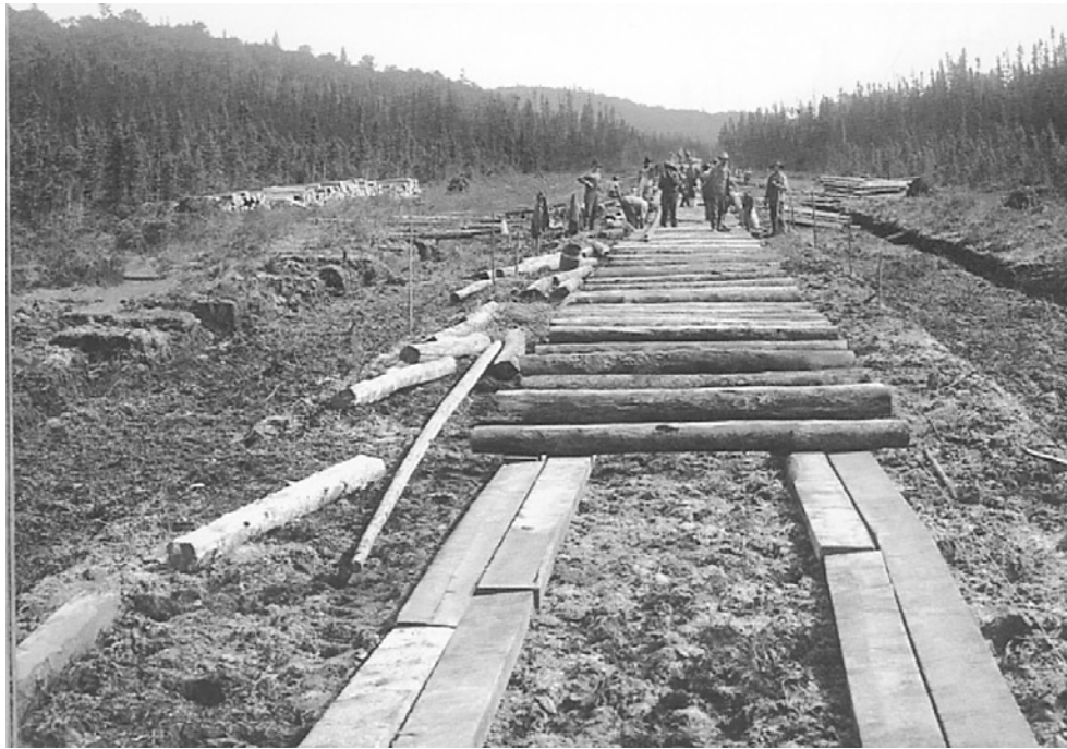
Figure 1.3 : Use of timber raft (corduroy) construction for an embankment over peat subgrade (MacFarlane 1969).
