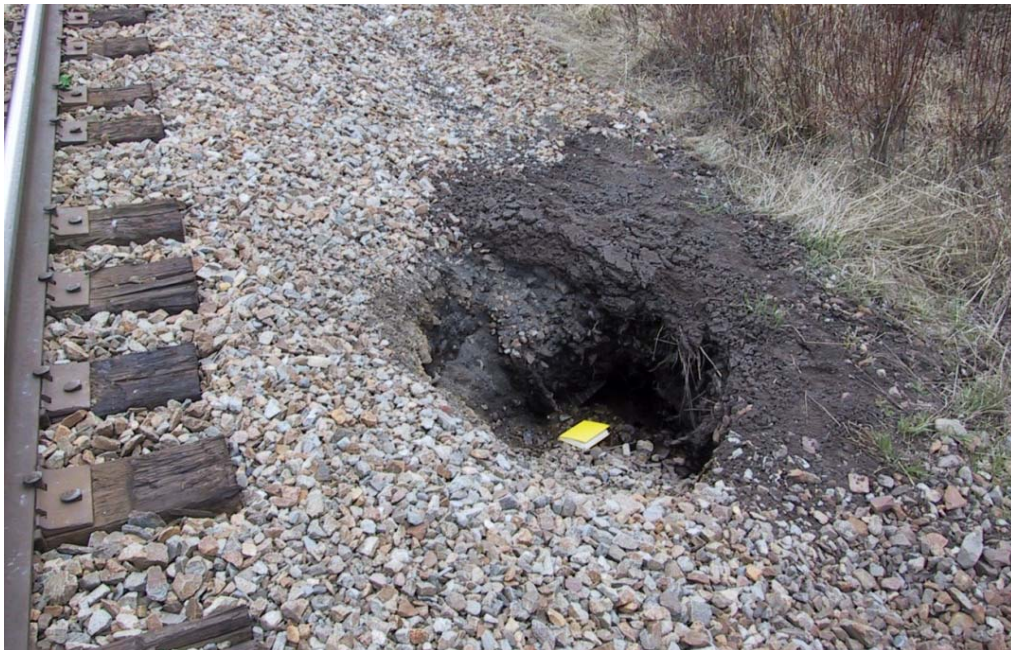
Figure 2.15 : Examples of large pumping features common in embankments over peat foundations (Moyie Subdivision Courtesy of CP).
